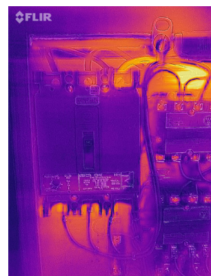
Identify electrical faults
